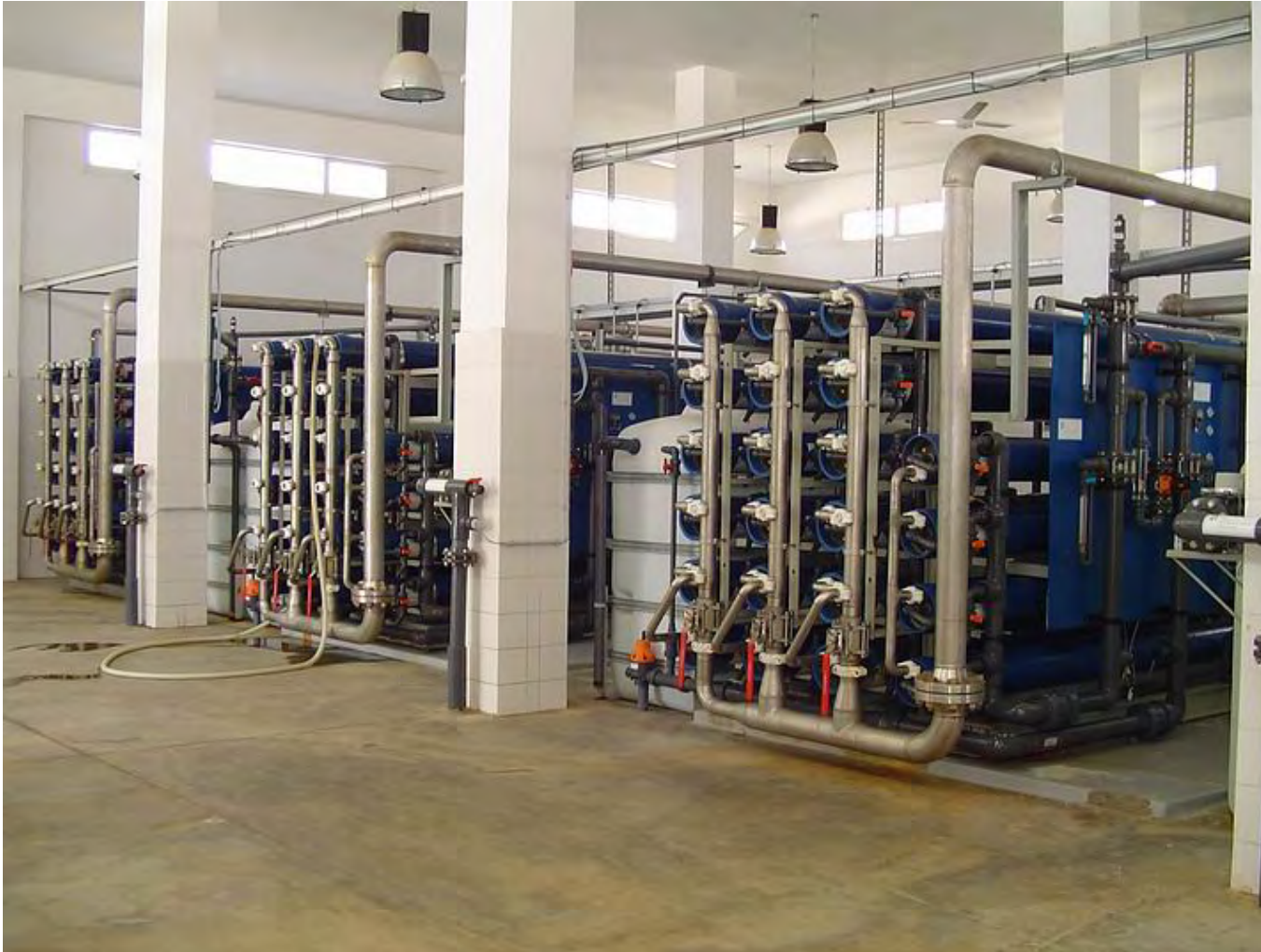
Seawater desalination plant, 3 x 1.000 m 3 /day (total 11x1.000 m 3 /d), Sharm El Sheikh, A.R.E.
