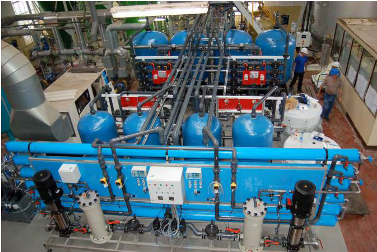
Double RO (2x20 m 3 /h), iron and manganese removal unit - Processwater treatment
