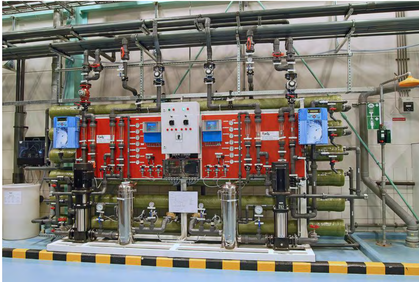
Nanofiltration 2 x 20 m 3 /h, Process water treatment
