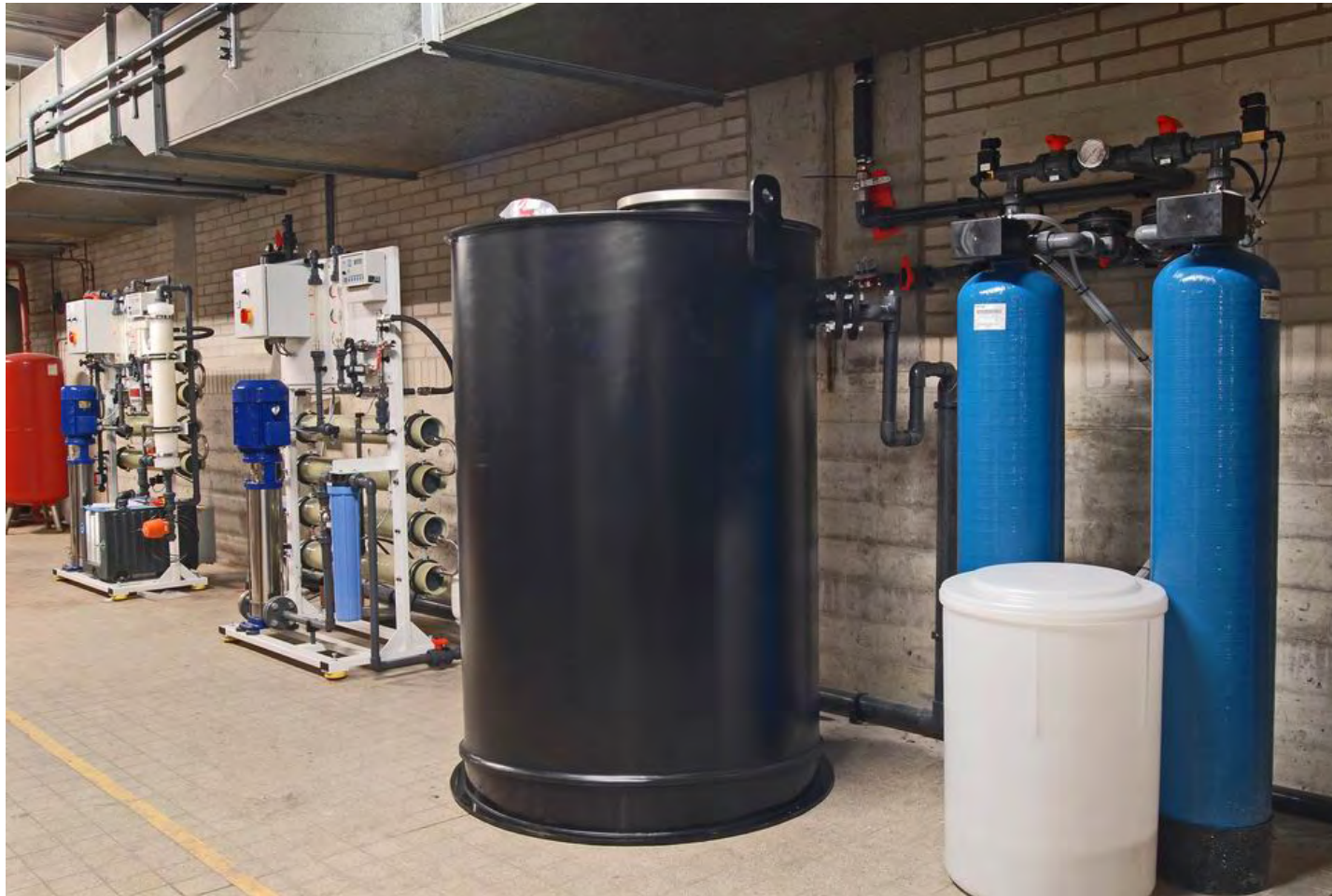
RO system and duplex softener, Hospital Rotterdam
