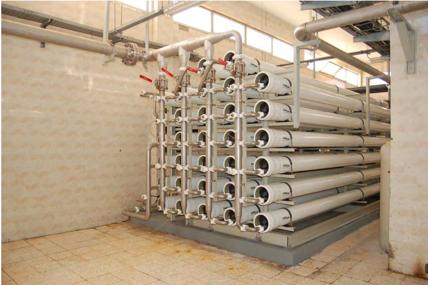
Seawater desalination plant, 1.500 m 3 /day (total 6.000 m 3 /d) , Sharm El Sheikh, A.R.E
