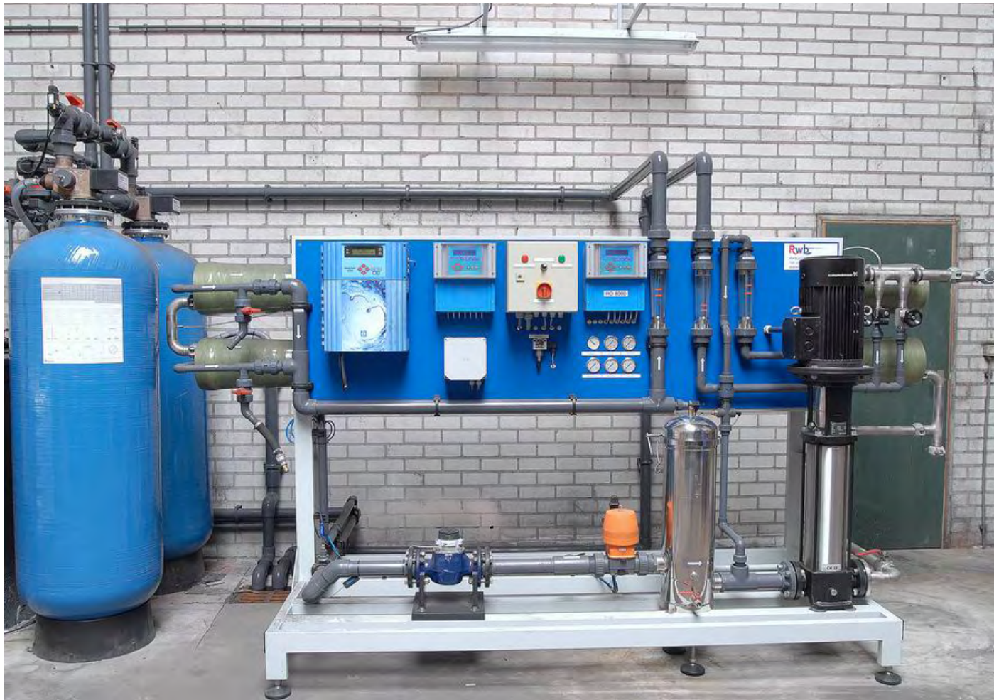
RO- 5 m 3 /h & Duplex softener
